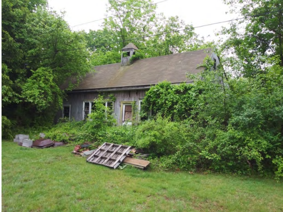
View of shed on property looking east taken by Vincent OBrien on May 28, 2020
